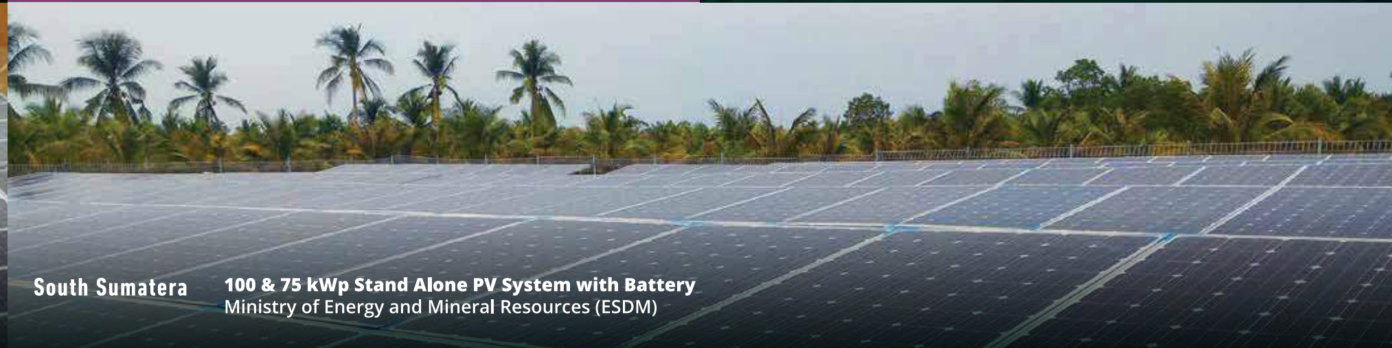
Gorontalo - South Sulawesi 100 & 15 kWp Stand Alone PV System with Battery Ministry of Energy and Mineral Resources (ESDM)
